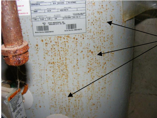
Rust on the outer shell of the water heater
