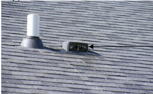
Lint at exterior discharge of dryer vent
